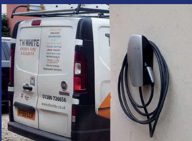
Electric vehicle charging
