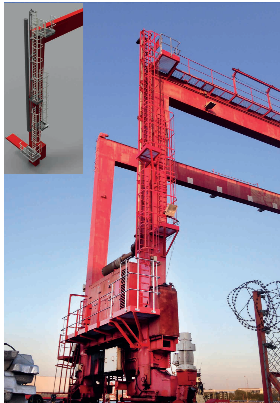
Job done! The access platforms, ladders and connections that T H WHITE Projects added to the Chinese-built crane gantry are now in place to provide a secondary personnel escape route. This project illustrates the flexibility of T H WHITE's fabrication and installation services. The 3D visualisation for the project is inset.
